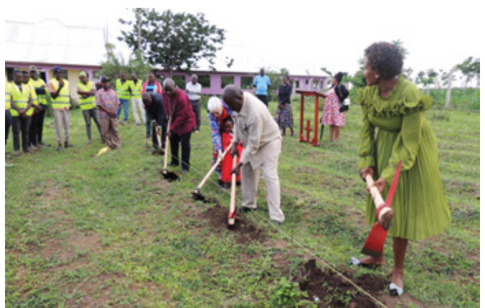
Bishop Dr. George Okoth lead a Ground breaking at shalom primary school for the building of new duplex staff house.
